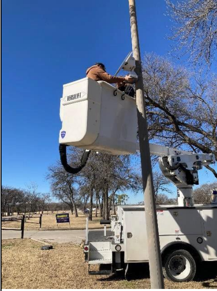
Figure 3. Pod Installation – Luna Vista Golf Course (January 24, 2025)
