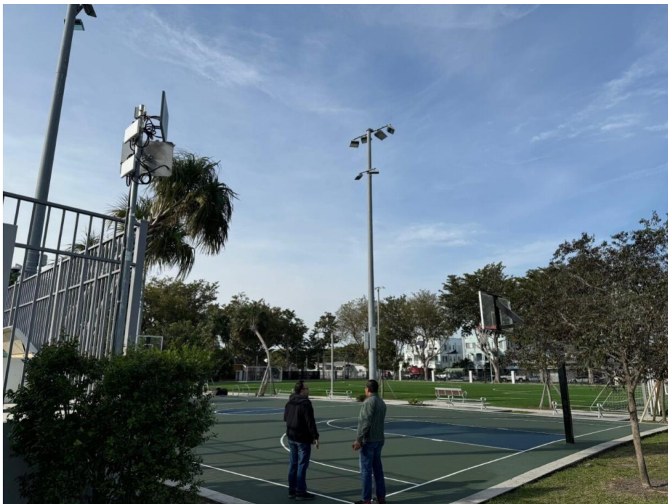
Figure 11: Shenandoah Park Wi-Fi installment (continued) at basketball courts.
