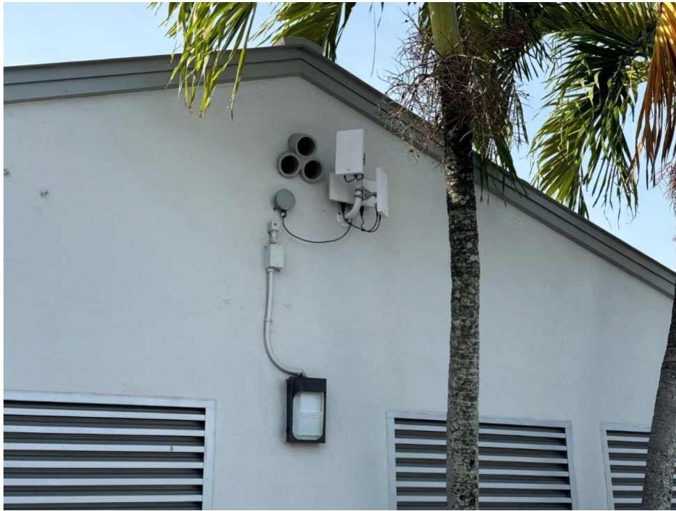
Figure 10: Shenandoah Park Wi-Fi installment.
