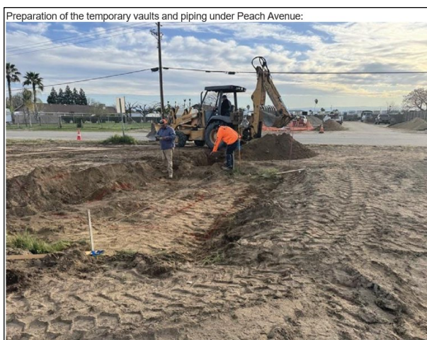
Figure 2-23, Malaga County Water District, Groundwater Well
