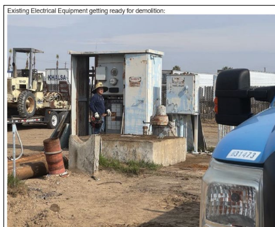
Figure 2-22, Malaga County Water District, Groundwater Well
