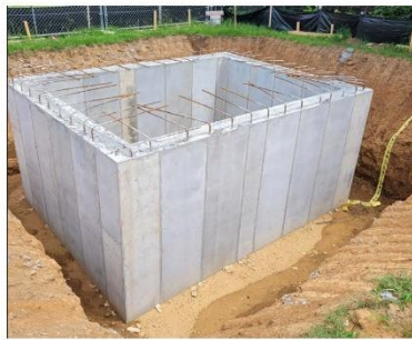
Surge tank for the new Douglass Pool
