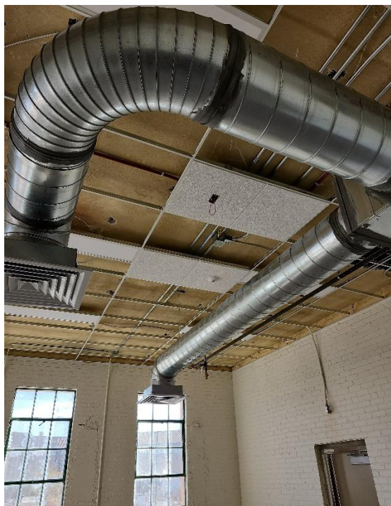
Curley School Gymnasium updated ductwork. Photo by Pima County Project Design & Construction.
