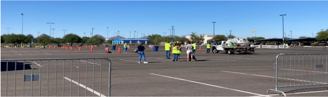
Kino Stadium District renovated parking lot. Photo by Pima County Stadium District.
