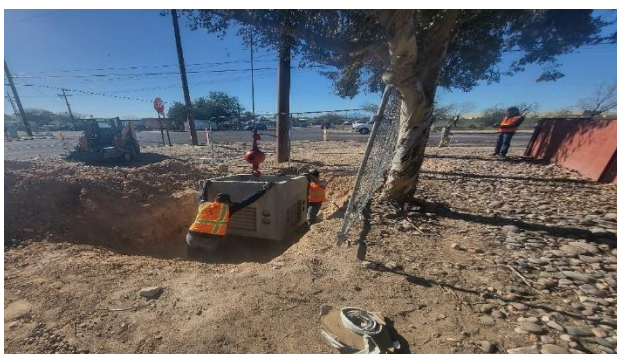
Fiber optic conduit infrastructure. Photo by Pima County Information Technology.
