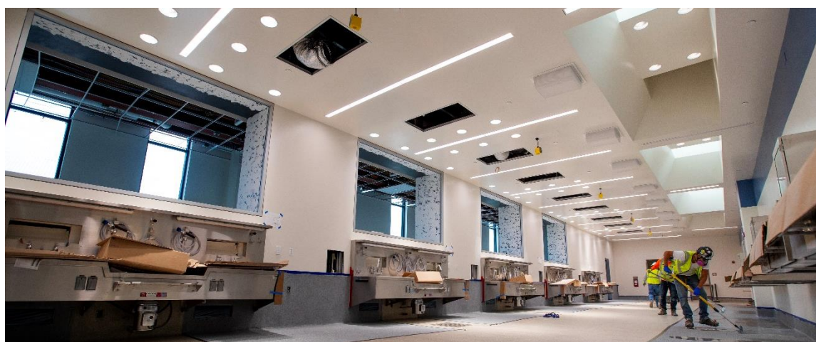
Office of the Medical Examiner autopsy area. Photo by Pima County Project Design & Construction.
