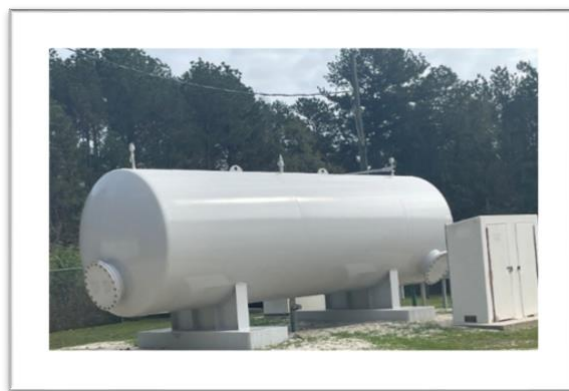
Hydropneumatic Tank Installed
