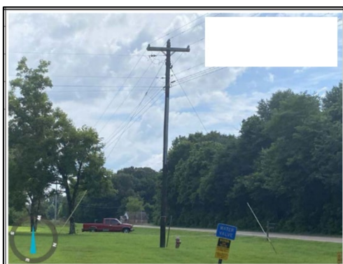
View of overhead lines, a splice case and a drop hut
