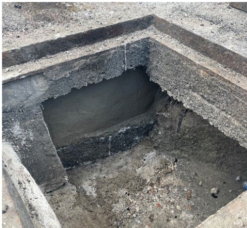
Town of Occoquan (440-410): Closed connection in the northwest inlet
