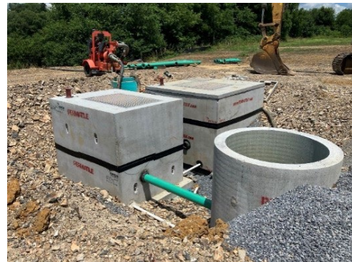
Washington County Service Authority (440-237): Halls Bottom Road Pump Station.
