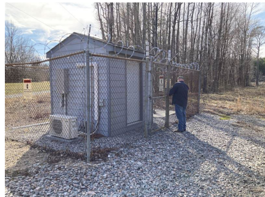
Cabinet in Dinwiddie County project with ISP, RuralBand
