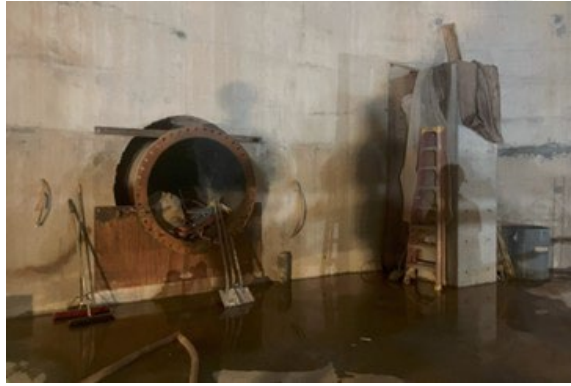
Alexandria Renew Enterprises (440-101): Bottom of drop shaft/tunnel dewatering pumping station
