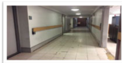
BROKEN AND CRACKED TERRAZZO TILES IN CORRIDOR C131
